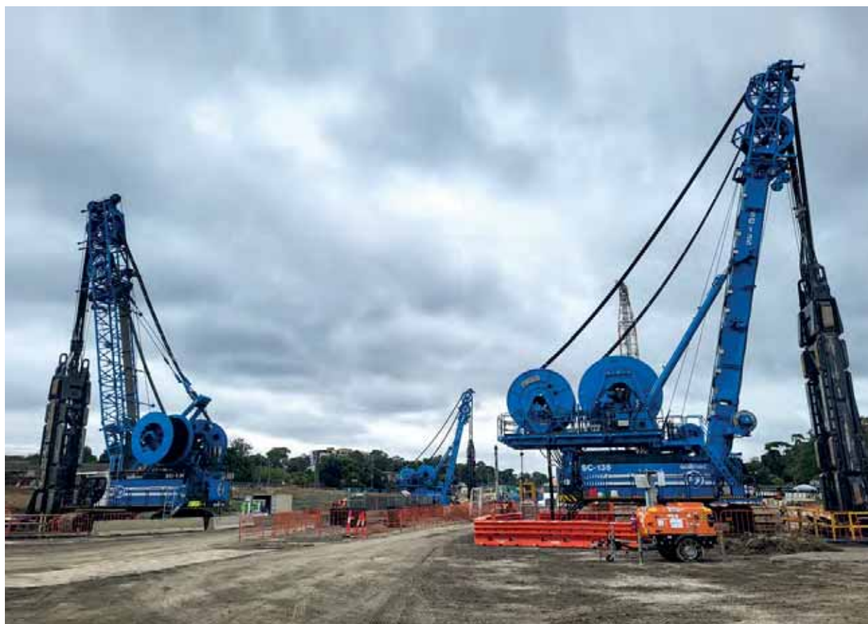
Soilmec hydromill model SC-135 "Tiger", at work in jobsite North East Link | Melbourne, Australia
